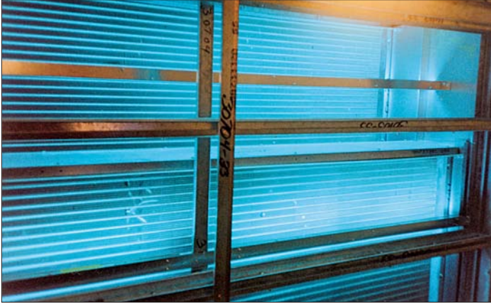
FIGURE 2. UV light in AHU applications can be used to control biological growth on cooling coils. (Photo courtesy of Steril-Aire.)
